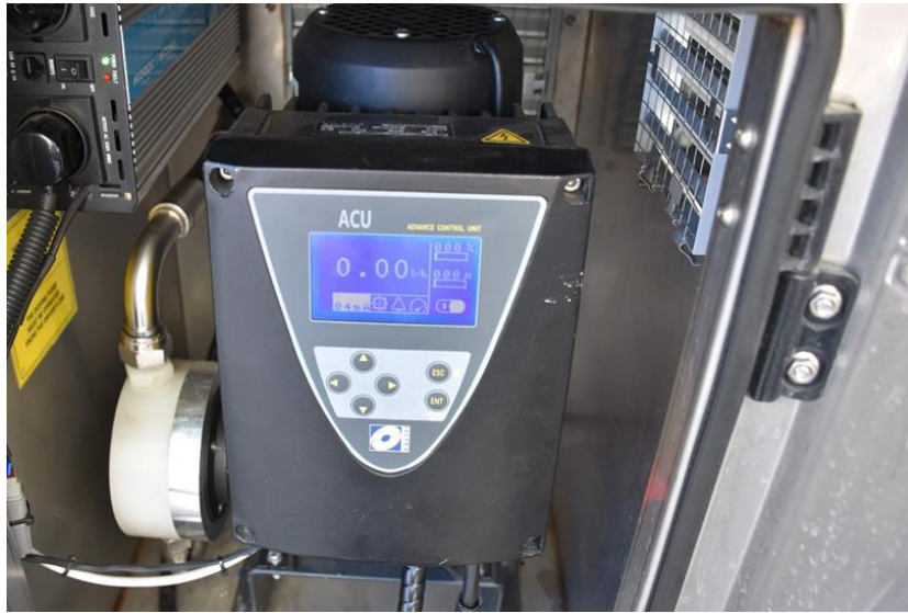
Detail showing the dosing pump for water-sanitizer mixture
